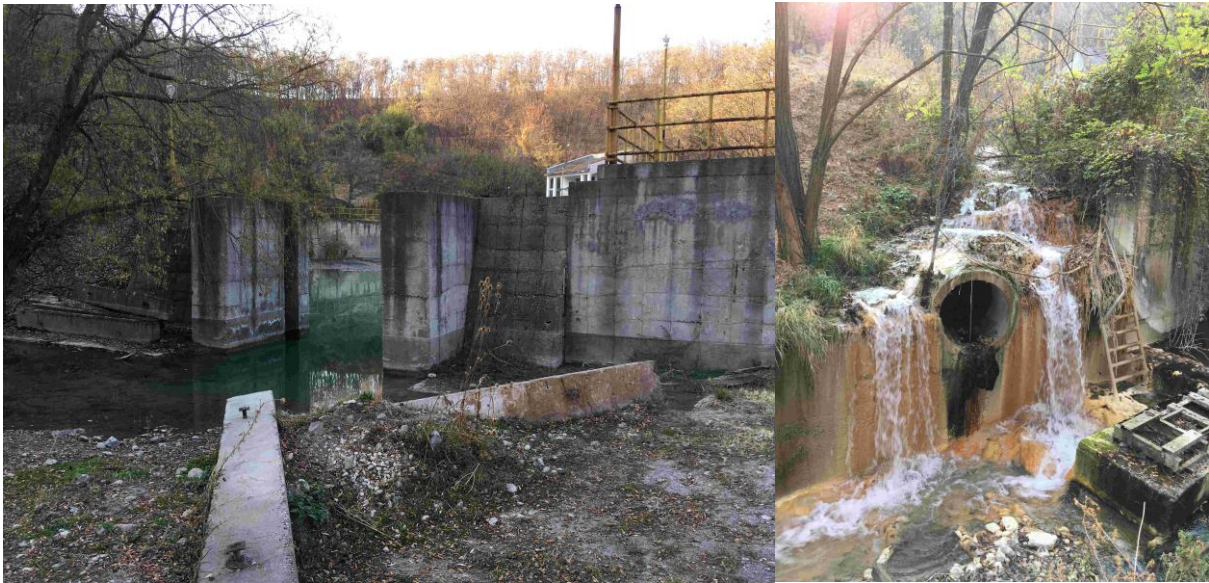
Figure 2. Uncontained water at the lower equalizer facility, and overflow of water from the storage area into a concrete channel
