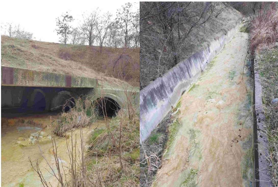
Figure 3. Concrete channel downstream of the lower equalizer facility as it re-emerges after flowing underneath the road, and small channel further downstream
